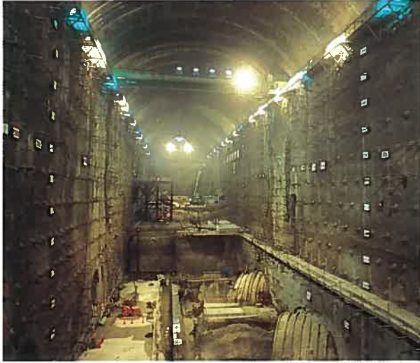
Sabigawa Power Station
