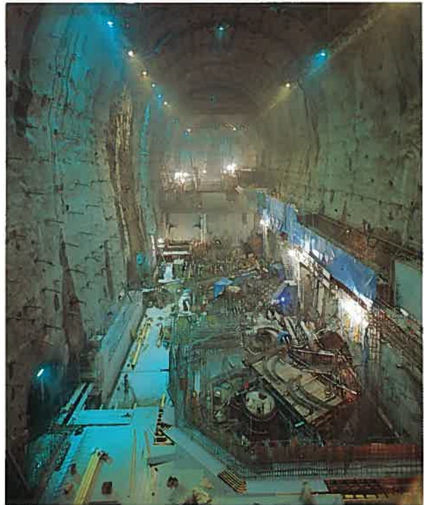
Imaichi Power Station
